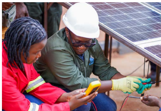
Two female experts in solar technology take readings of a solar module.
